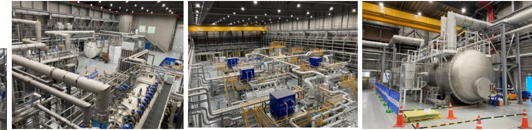
Cold box Warm compressors LHe Dist. box
